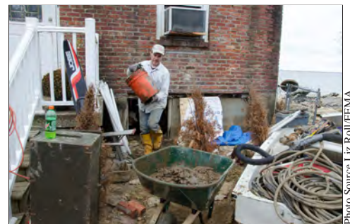
Joe Barry, a volunteer from the United Methodist Committee on Relief, helps a homeowner clean after Hurricane Sandy washed away exterior walls and completely filled the basement.
